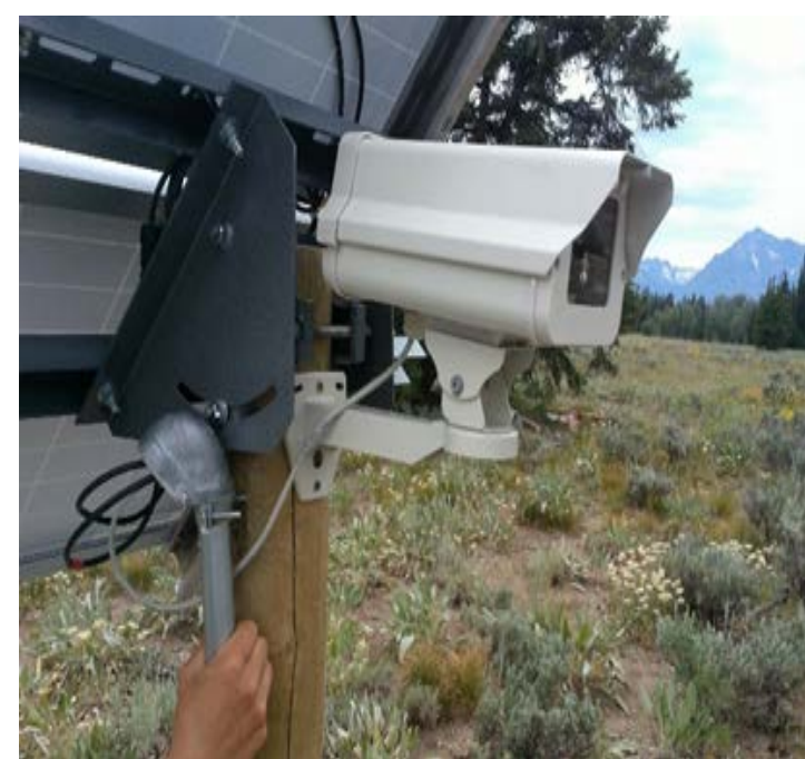
Camera and solar panel showing cables looped prior to entering conduit to allow for condensation or precipitation to drip outside of conduit. We later used a zip tie to secure them together more tightly.
