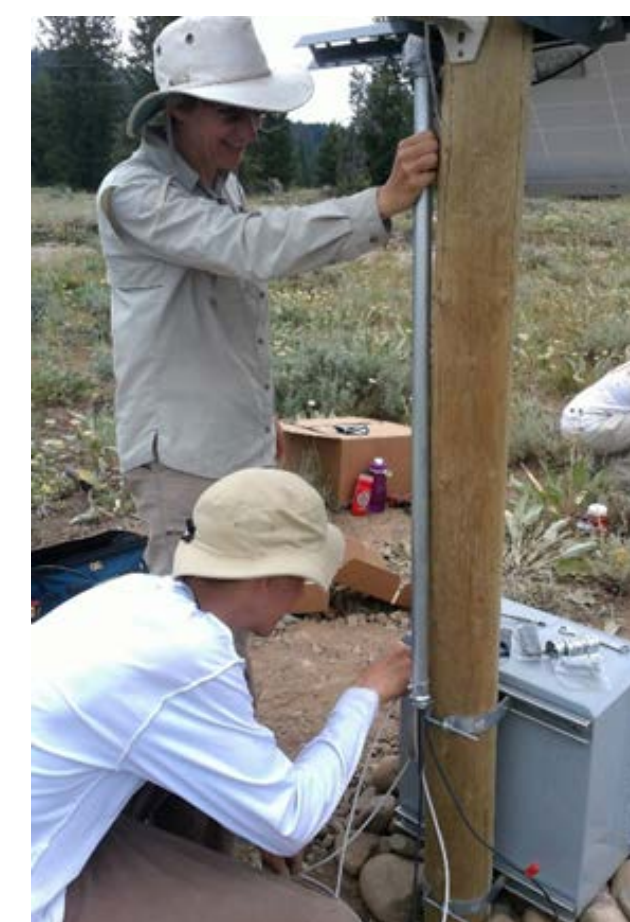
Audrey and Joe attaching conduit to post and feeding cables from conduit into box.
