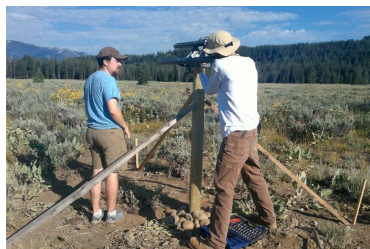
Joe and Daniel affixing hardware that will hold solar panel to post. Note: wooden stakes had been used to prop up pole while cement dried.
